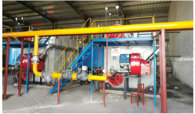
2018.09.20 河南周口郸城天豫薯业2台10吨30毫克低氮冷凝锅炉 2018.09.20 2 sets of 10t/h low nitrogen condensing boilers in Zhoukou Tianyu Potato Industry co.,Ltd
